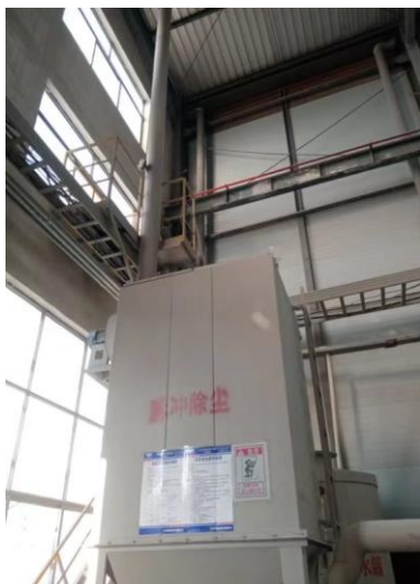
1#布袋除尘器排气筒及采样孔
